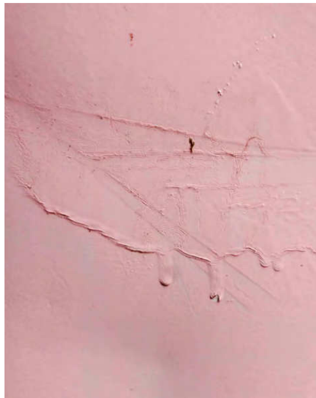
Figure 2 Detail of Flause . Drips visible in the surface structure of the paint indicate a lack of careful paint application.
