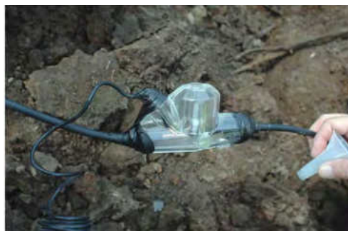
Figure 10b Plastic housing is used as a cable connection.
