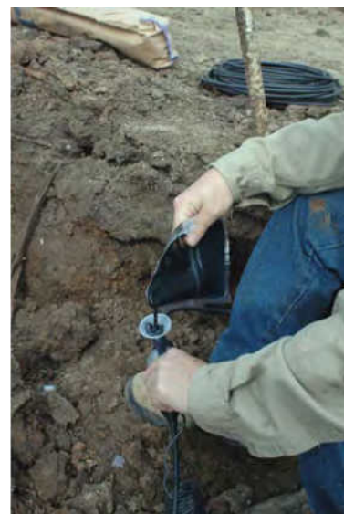
Figure 10c The cable connection housing is filled with a bituminous material to make the cable connections waterproof.
