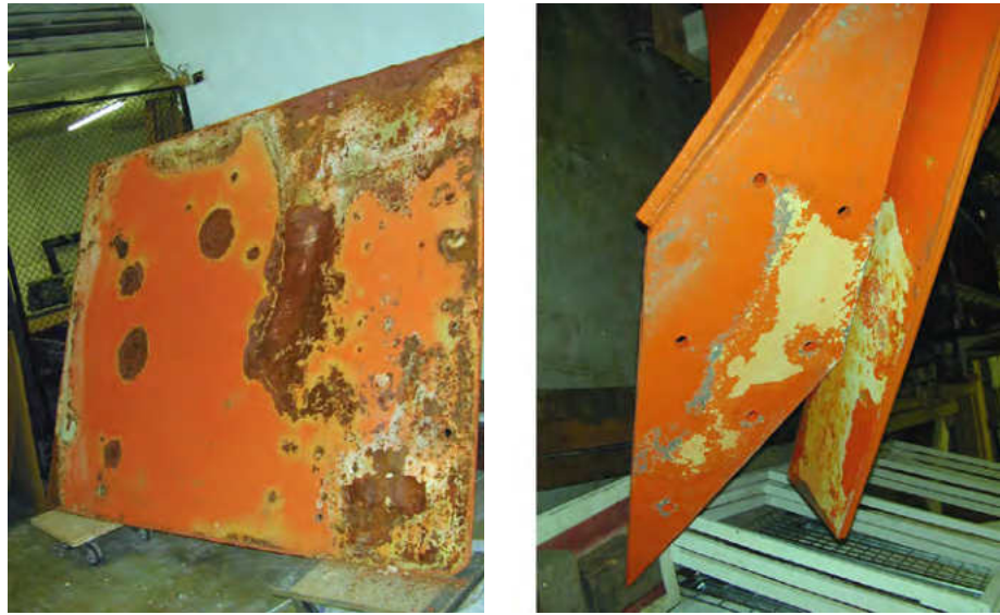
Figure 9 (Right) Bottom surface of the base plate, showing heavy rust and missing paint. (Far right) Detail of the contact area between steel beams, showing heavy rust and missing paint.
