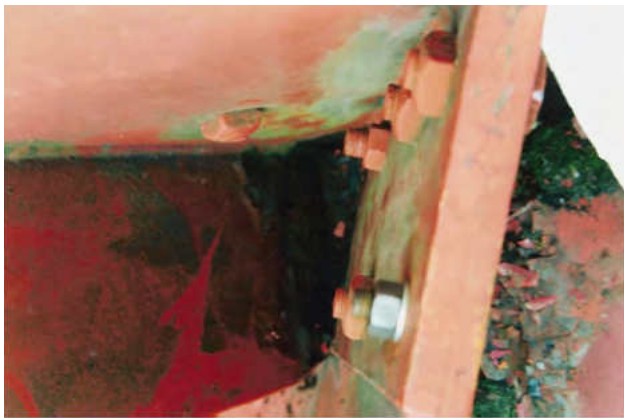
Figure 9 In the corners of the sculpture, pockets form where water can collect, leading to corrosion. © 2014 Calder Foundation, New York / Artists Rights Society (ARS), New York. © ZMK, Hannover 2003.
