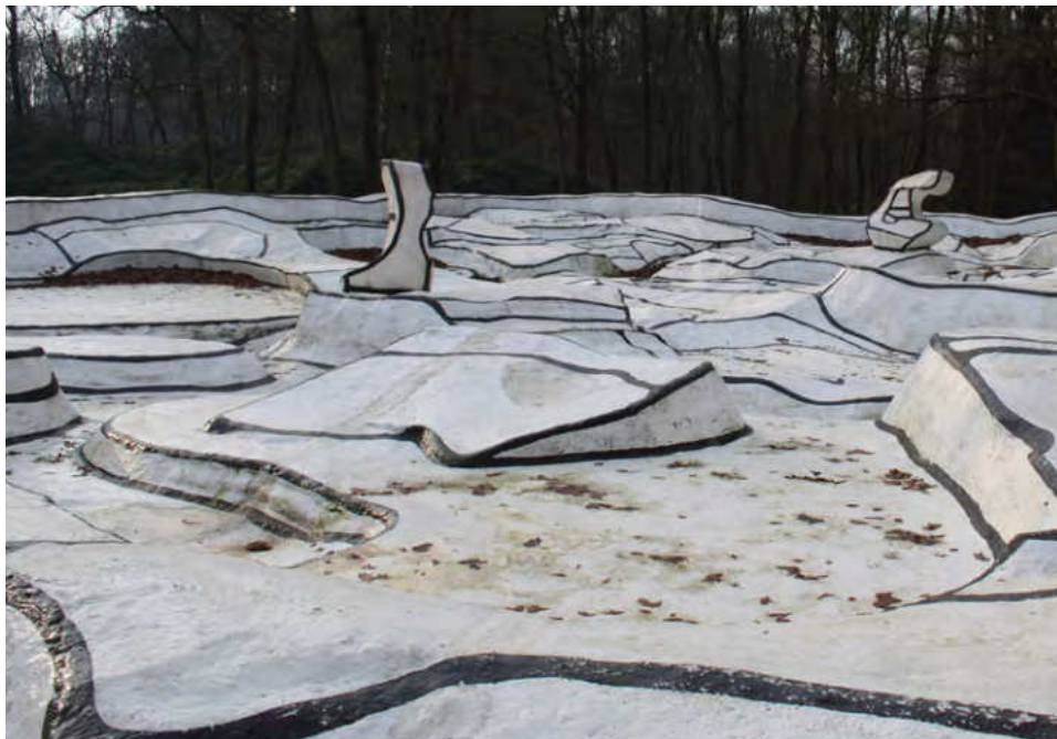
Figure 9 View of Jardin d'émail , showing numerous local paint repairs. Photo: Frederike Breder, 2012.
