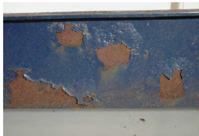
Figure 2 Detail of One for Bristol , indicating paint loss and corrosion in 2010. © The Artist's estate.
