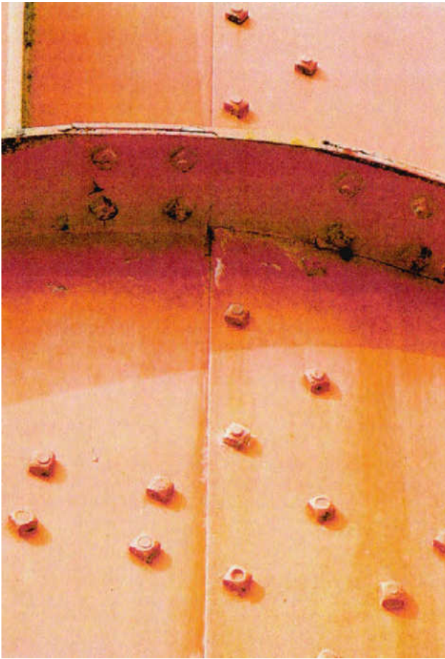
Figure 7 Photo of the west-facing side, showing rust and runs. © 2014 Calder Foundation, New York / Artists Rights Society (ARS), New York. © ZMK, Hannover 2003.
