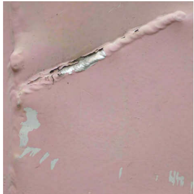
Figure 4 Detail of Flause , showing flaking paint caused by expansion of the aluminum underneath.
