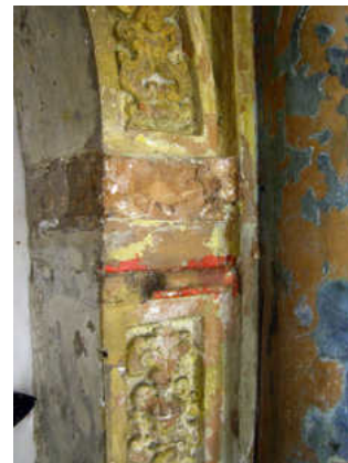
Figure 8. Incise lines are visible marking the position where the frieze moulded frieze decoration should be adhered. © IMC-DGPC
