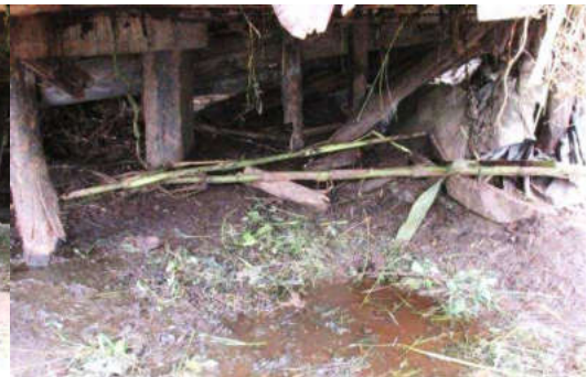
Fig. No. 2.4.4.1 Shed in bad condition- littered waste
