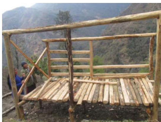
Fig. No. 2.4.3.2 Laying the wooden planks with appropriately so the goat's leg will not pass from holes
