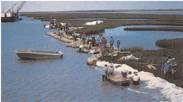
Erosion control efforts along the Intracoastal Waterway at Aransas National Wildlife Refuge © TPWD
