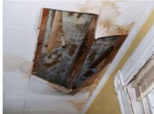
Fig. 75 Roof construction damage by mould
